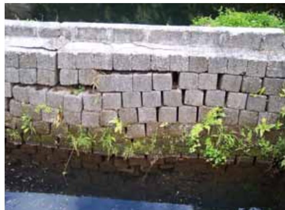
Wall conditions of the Holding tank at Avana Intake
