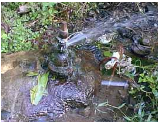
Lack of maintenance of network
