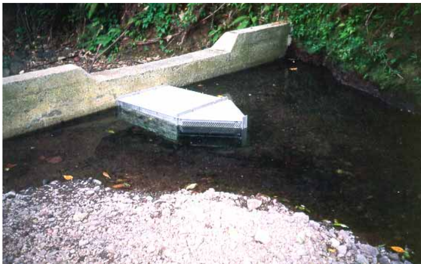
Concrete encased intake mouth to exclude leaves and debris
