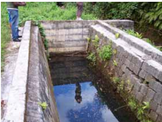
Holding tank at Avana Intake
