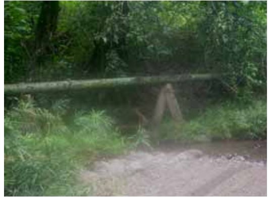
Pipe transporting water from Avana Intake to the distribution main
