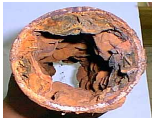
Internal condition of pipes affects water quality.
