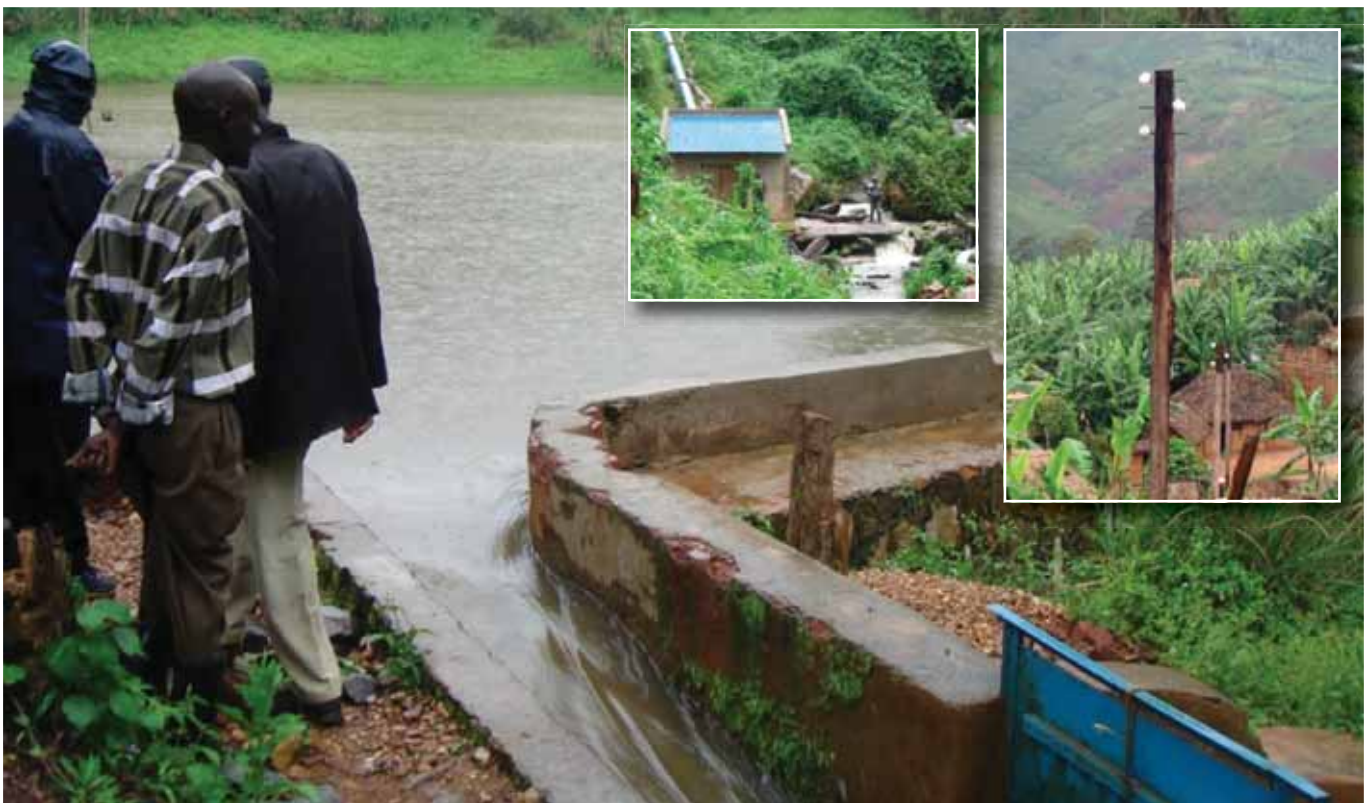
Hydro-electric station (37 kw) serving TCCB, the radio station and village of Kasugha. A dam with sluice feeds a gravity drop pipe into the turbine station, generating the electrical current. From there, through several transformers, the current reaches the TCCB more than 4 km distance, and also is sent to the village of Kasugha, where it drives public lighting and several micro-projects.
